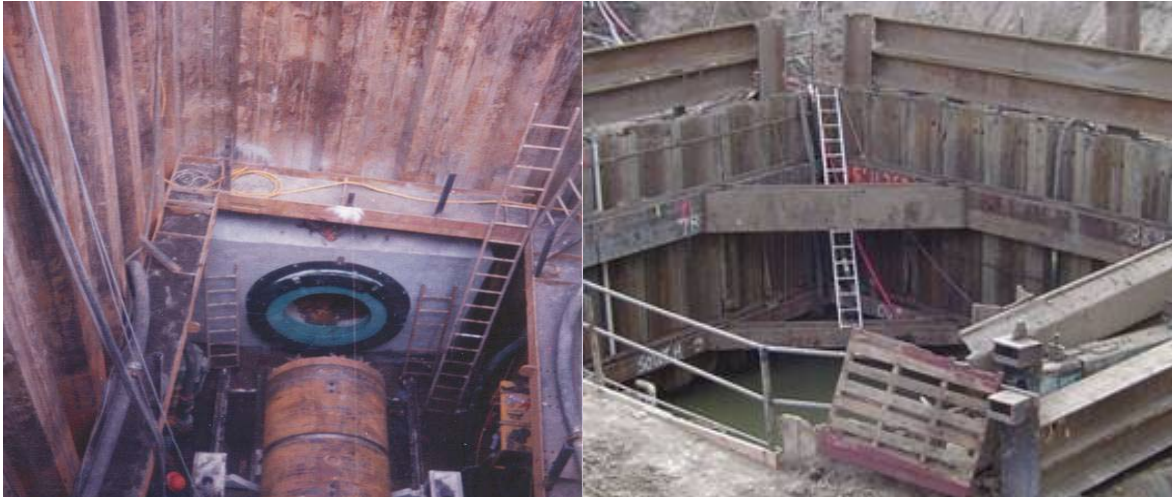
Figure 7. Sheetpile jacking shaft prepared for launch of the MTBM (left) and a shaft that flooded during construction with split interlocks allowing high inflow of water (right)
