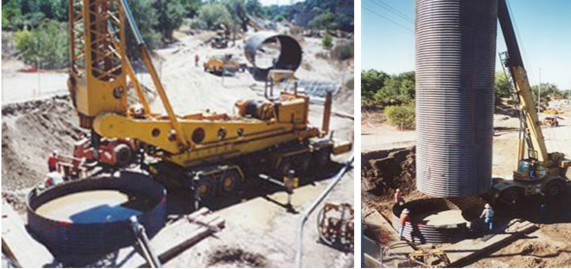
Figure 4. Large diameter auger-drilled reception shaft constructed for a microtunneled drive adjacent to a river
