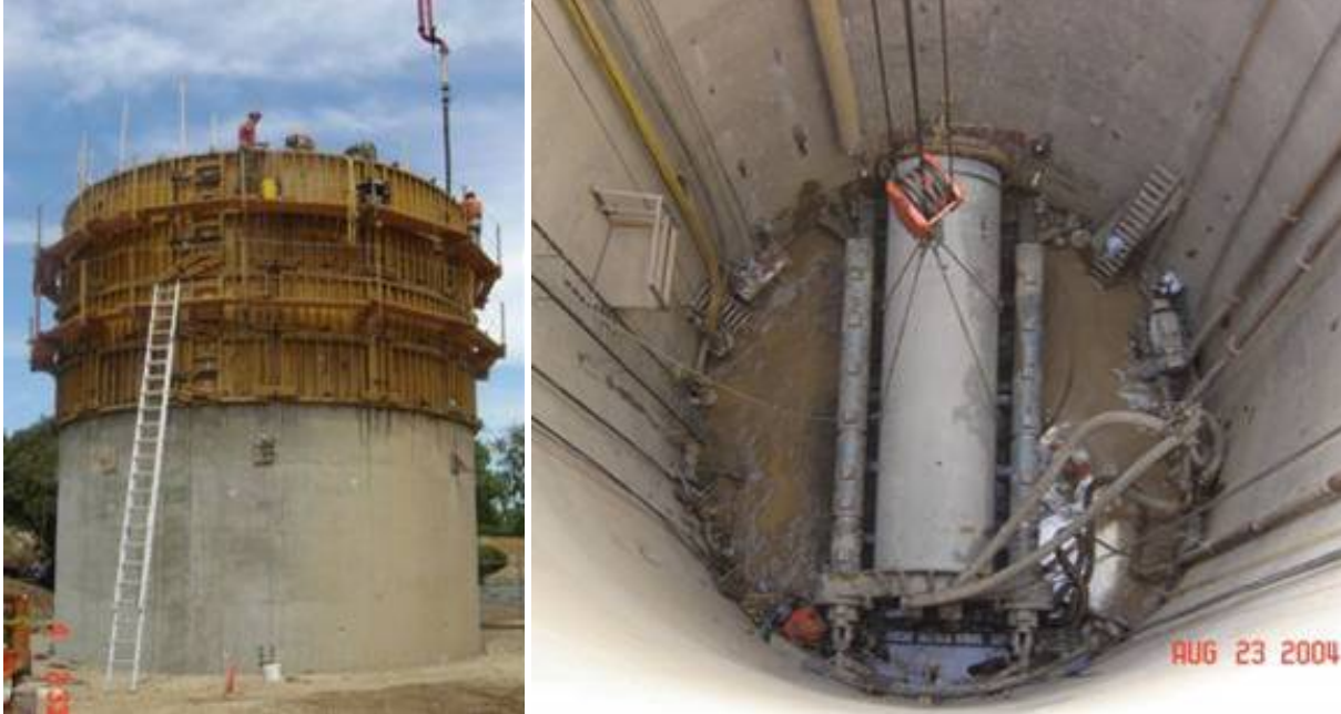
Figure 5. Concrete caisson shaft during construction (left) and being used as a jacking shaft (right) for river crossing projects
