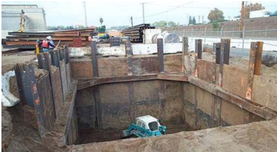
Figure 1. Soldier pile and steel plate lagging shaft used on an Interstate crossing
