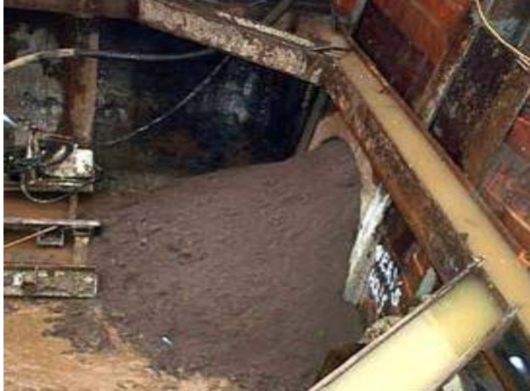
Figure 2. Loss of approximately 10 cubic yards of soil into the soldier pile and lagging shaft during cutting of portal for launch of MTBM
