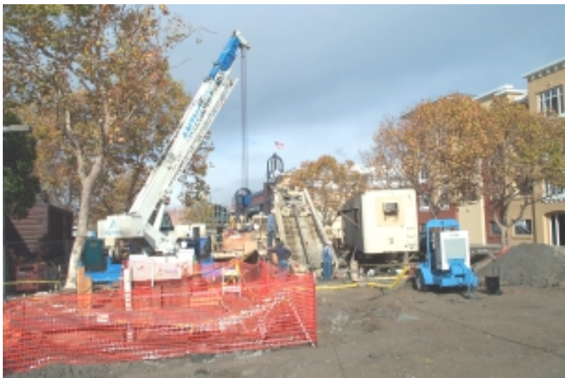
Figure 2 Rig-Side Equipment Layout -- Oakland
